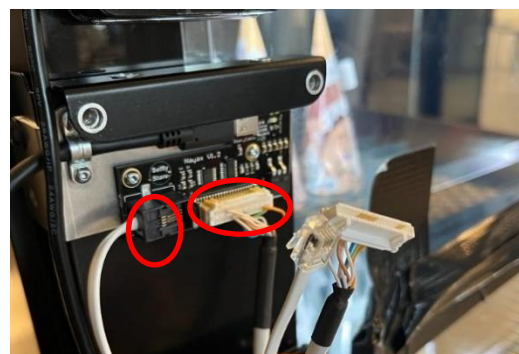
Cabinet with universal cabling
