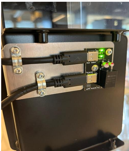
Cabinet with universal cabling
