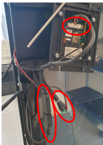
Cabinet without universal cabling
